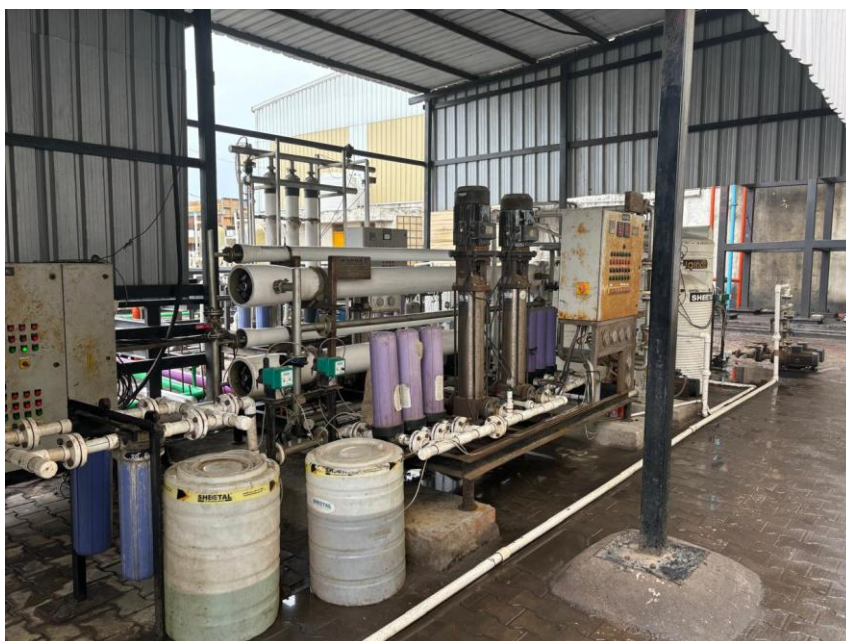
(Image 3; Water Flow Meters)
