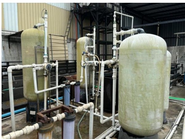
[Image 6; Filter Press (Sludge Water Extraction)]
