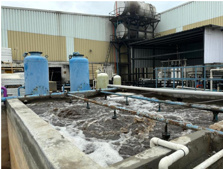
[Image 2: Sand Media Filter and Carbon Filter Plant (UF → Media Filter → RO)]
