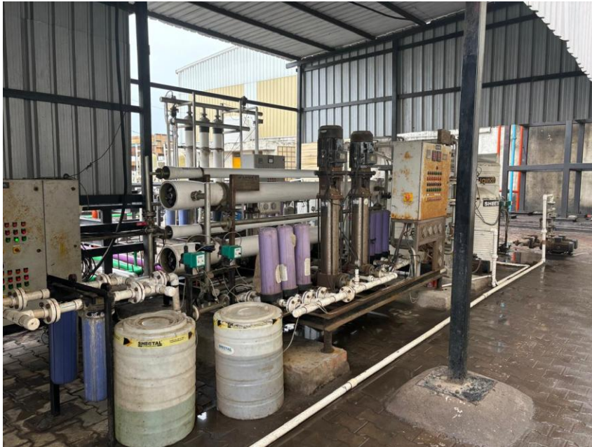
(Image 3; Water Flow Meters)
