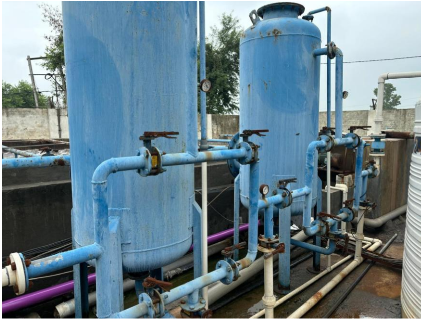
(Image 1; Reverse Osmosis Plant)
