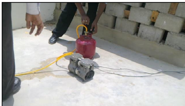
Figure 5 Gas cylinder and compressor
