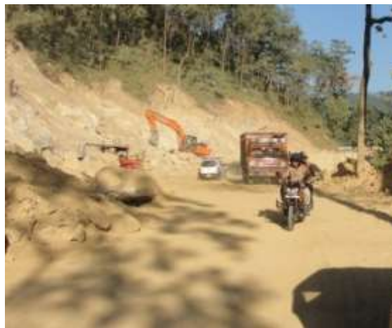
Fig 7:- Landslide prone access to Nainital Township.
