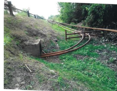
Fig. 2.3:- Gas flow station in Rivers State, Nigeria.
