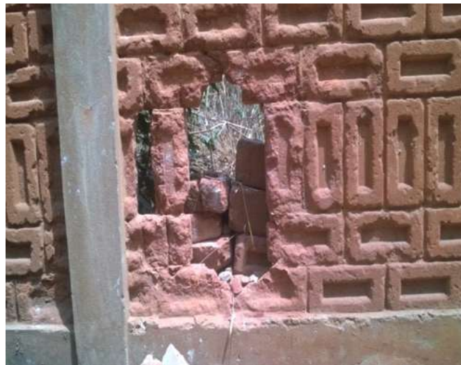
Fig. 3:- Example of wall decrepit and drilled.
