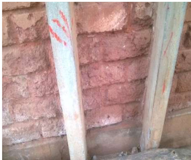
Fig. 4:- Example of crumbling wall.
