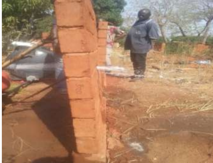
Fig. 12:- Drilling of the wall by the jet of water (dosage of 3 and 4%).
