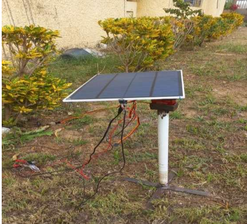
Figure 5:- Photocell solar panel with photoresistance and temperature sensor.
