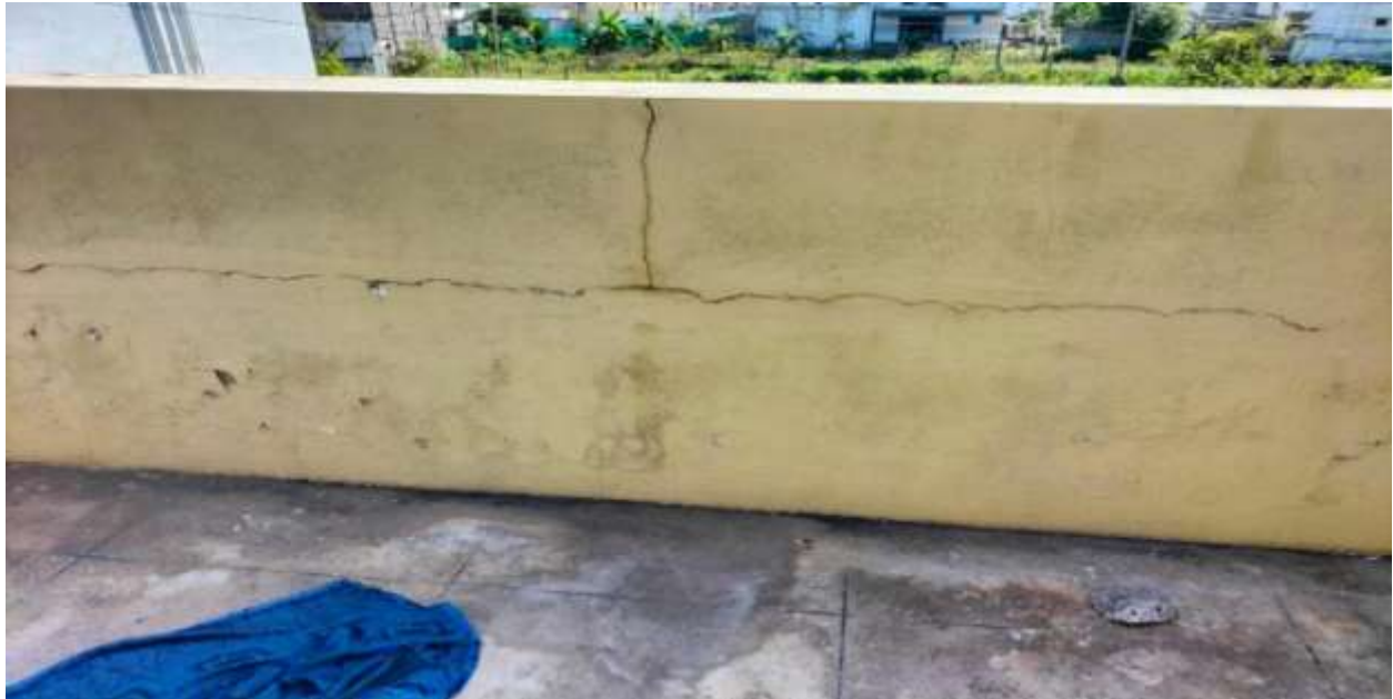
Crack Formation In Parapet Wall – Krishnagiri
