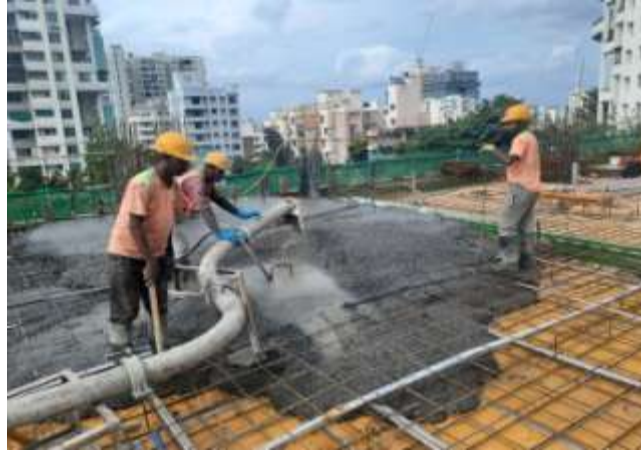
Figure 5:- Improper Bends Provided to Concrete Pipes.
