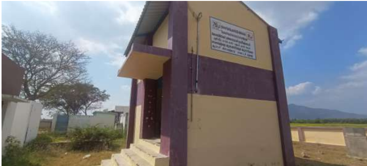
Figure 9:- Herbal Unit in Ambalathadi Panchayat, Madurai, lacking locks and proper compound walls for protection.
