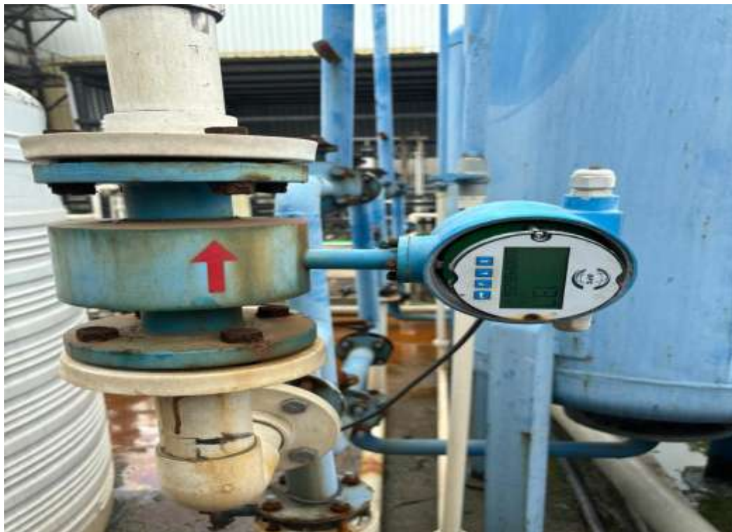
(Image 4; Physico-Chemical Reaction Chamber with Ferrous, Lime, and Polyelectrolyte Dosing, followed by Sludge Settler)
