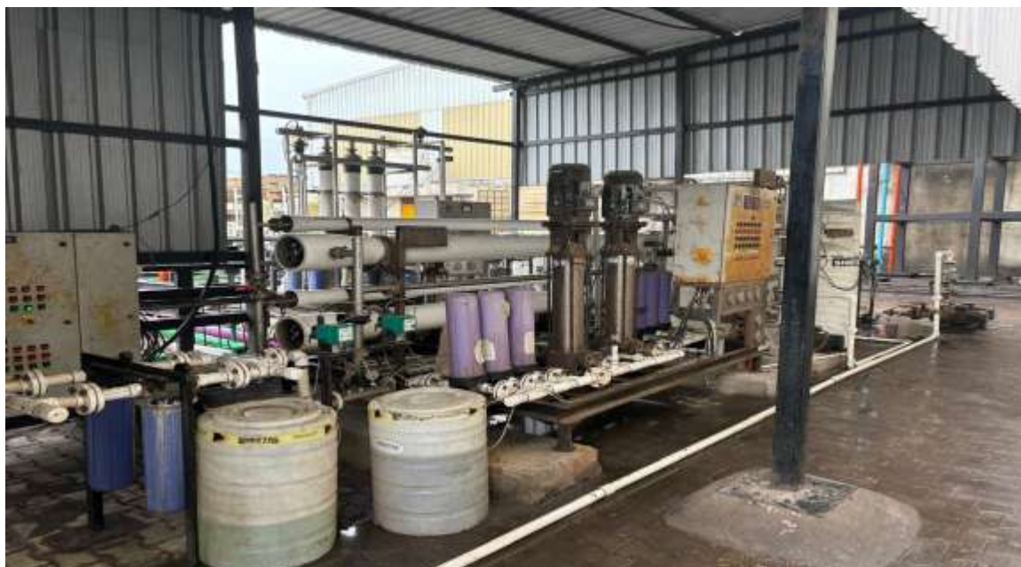
(Image 3; Water Flow Meters)
