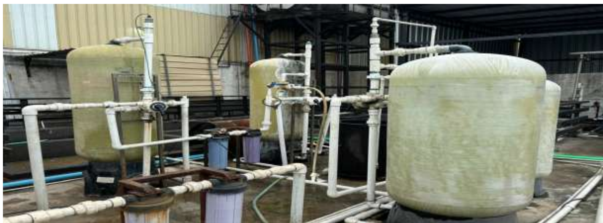
[Image 6; Filter Press (Sludge Water Extraction)]
