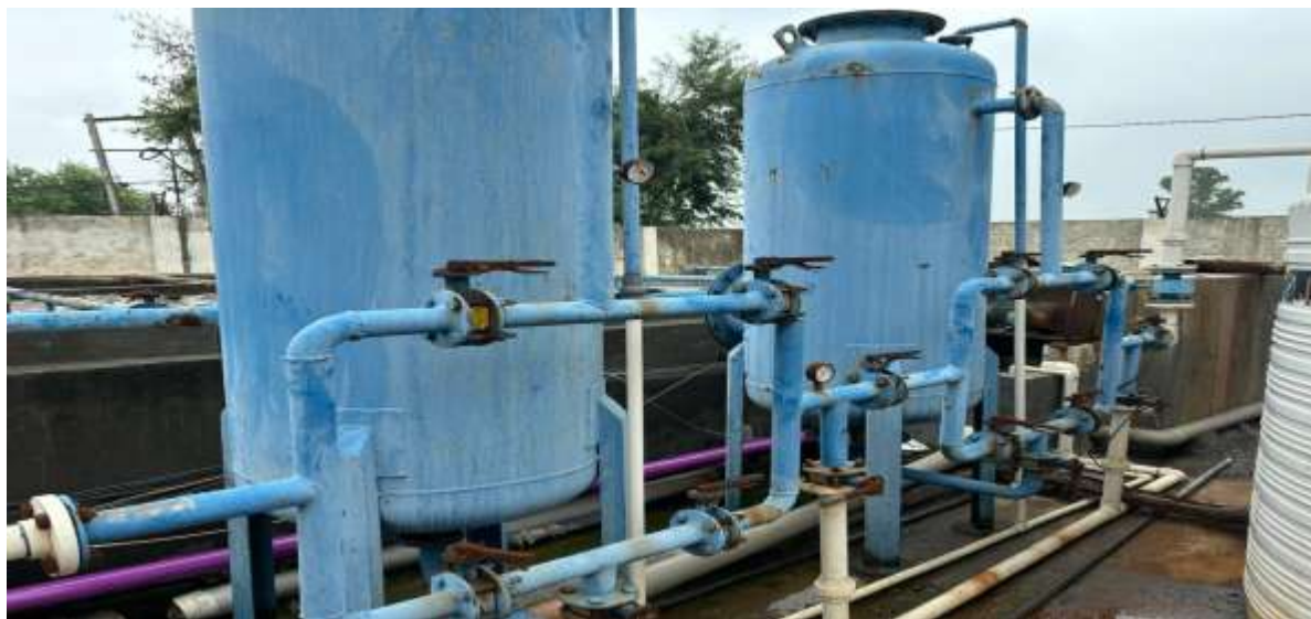
(Image 1; Reverse Osmosis Plant)
