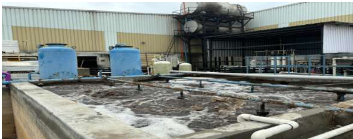
[Image 2: Sand Media Filter and Carbon Filter Plant (UF → Media Filter → RO)]
