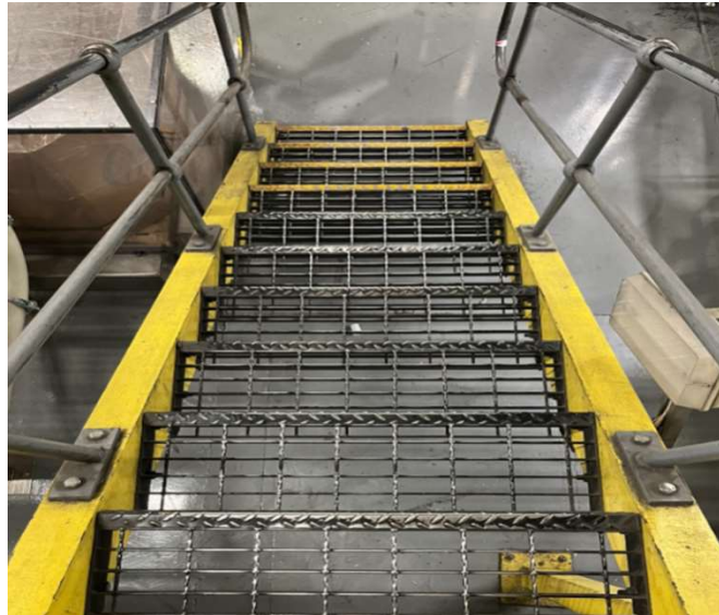
Figure 7. Improved visibility treatment applied to stairs in the bottling hall and Engineered Building Services area
