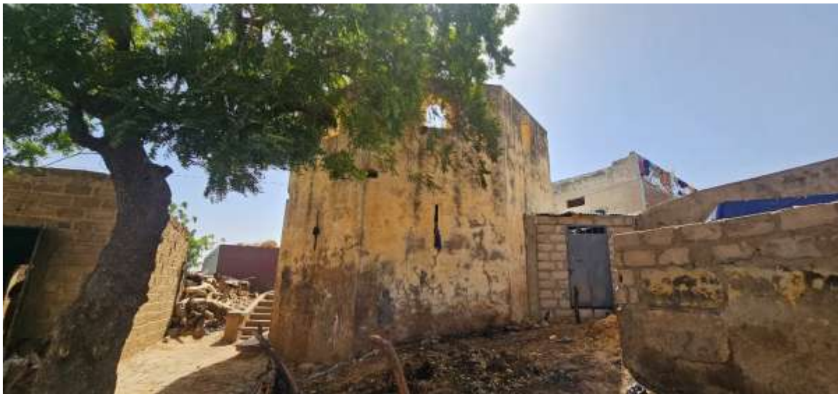
Fig.6: Tour Brue in deterioration
