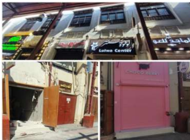
Figure 8: Signage, Façade, and Protection Quality Distortion
