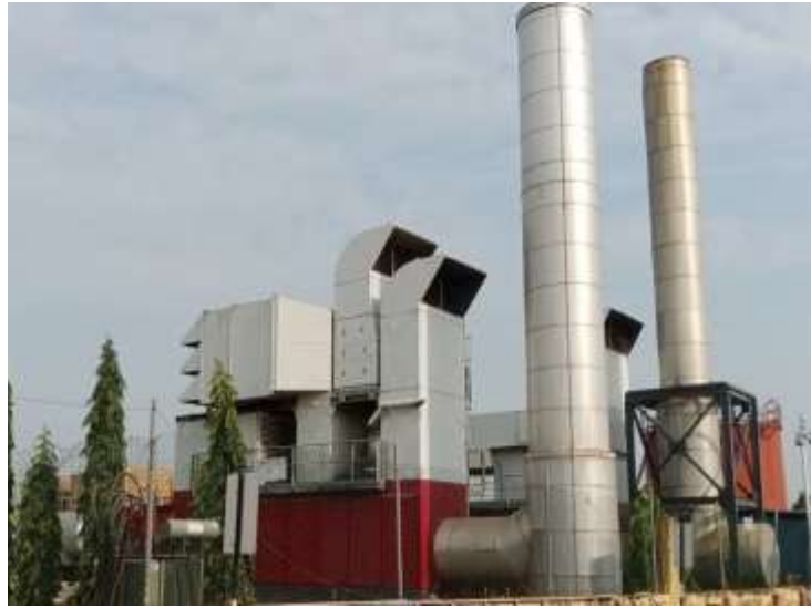
Figure1: Gas Turbine Power Generator GT1(5.2MW) and GT2(5.6MW)
