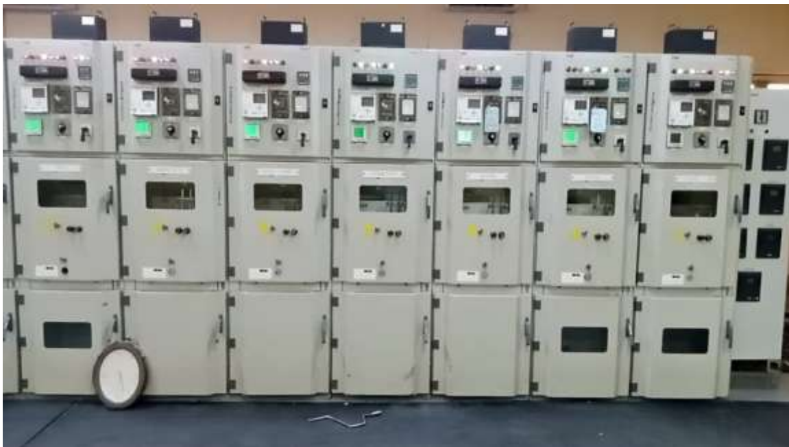
Figure 4: In comer feeder-2, 11KV Control panel and the six distribution feeders were installed.
