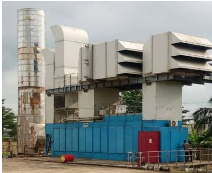
Figure 2: Gas Turbine Power Generators GT3 15MW
