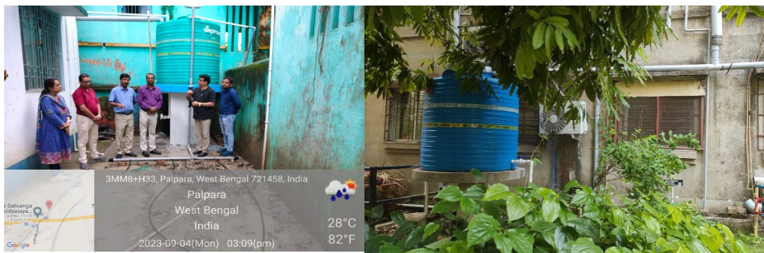
Installed the Basurtirtha Rain Water Harvesting Unit in Different Institution for Water conservation
