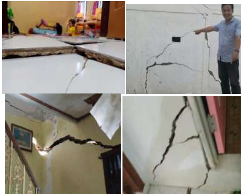
Figure 4:- Condition of Cracked Houses in Rafika 4 Housing Complex (source: https://sumsel.tribunnews.com/2020/ )
